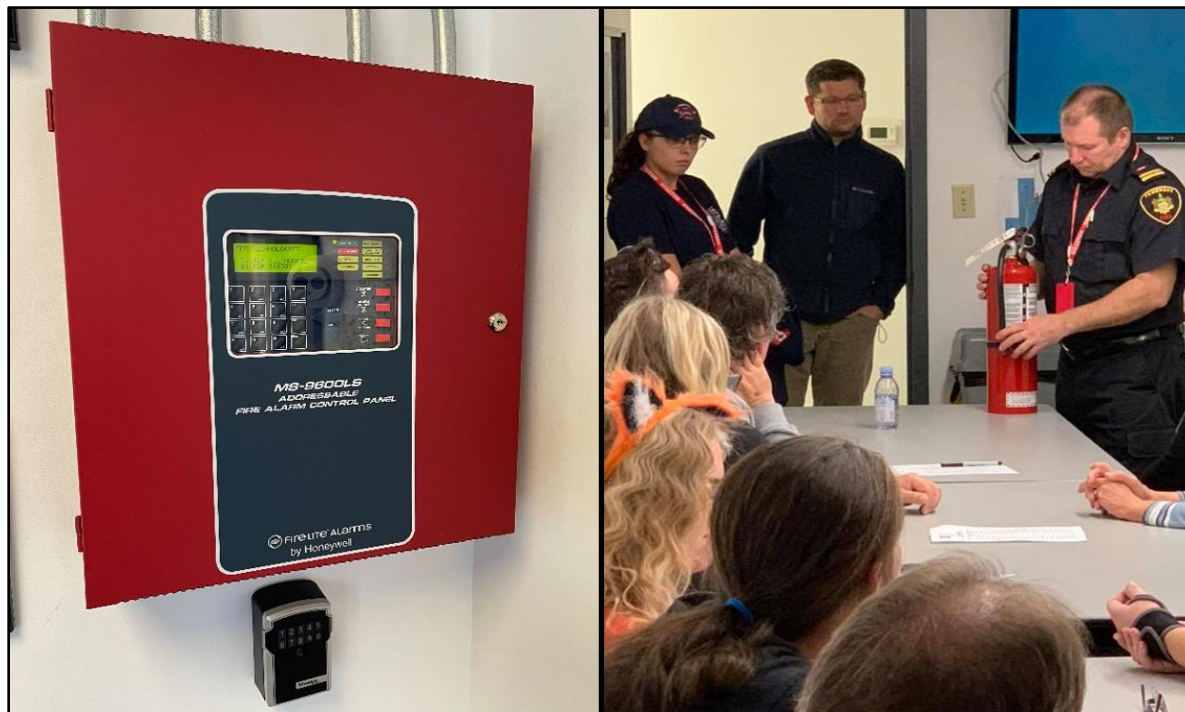
Figure 31: The SRBT facility includes a comprehensive suite of fire and life safety systems and components, such as the central fire alarm control panel (left). Members of the Pembroke Fire Department train SRBT employees on the use of fire extinguishers annually. A part of the training is shown from 2018 (right).
