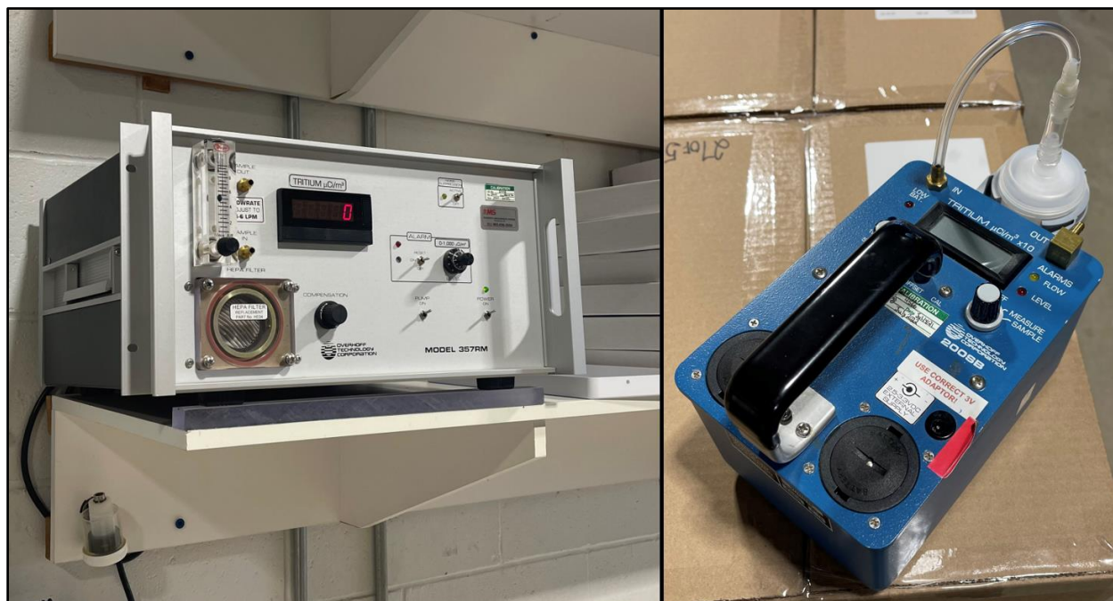
Figure 23: A tritium-in-air monitor (left) continuously samples air in the Shipping and Receiving Area, in order to alert staff in case of an upset condition. Beneath the monitor, a passive air sampler is mounted, to determine the lower-level, chronic concentration of tritium in the working environment over time. Portable tritium-in-air monitors (right) are also available for use throughout the facility.
